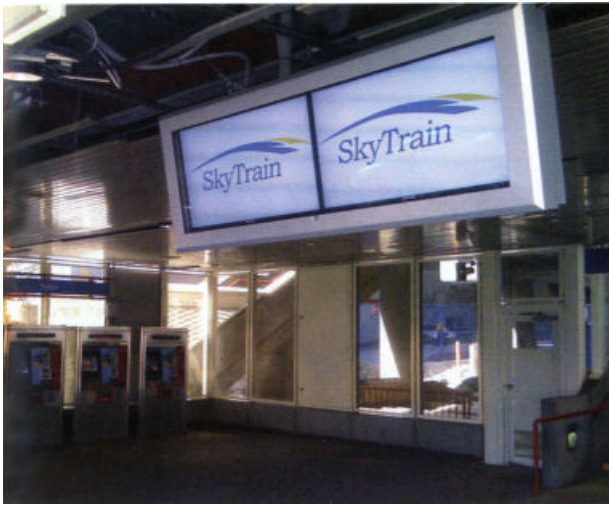
The new Station Entrance Emergency Information Panels (SEEIPs) are installed in locations where they can alert passengers before they buy tickets.
